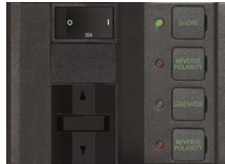
Circuit Breaker Source Selection
